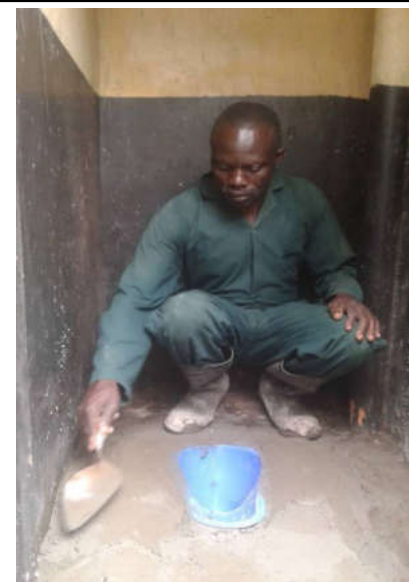
Some of the funds went towards renovation of latrines. Photo by IRC Uganda.
